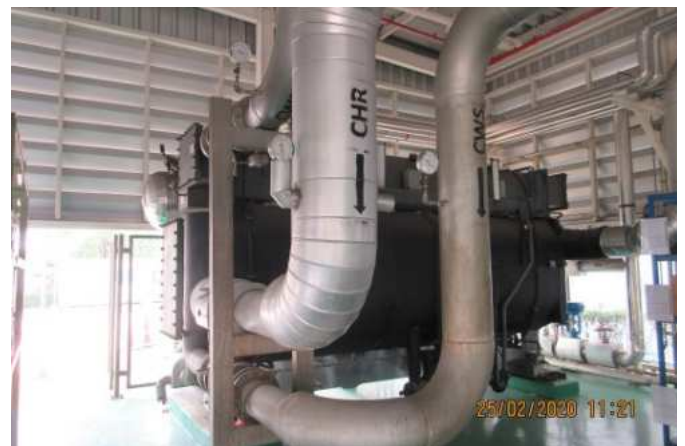
Absorption Chiller Production A
